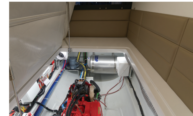
The hybrid eco drives fit neatly under the cabin sole boards
